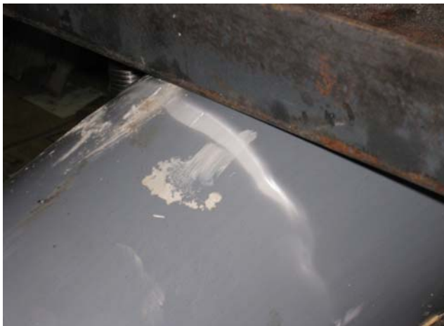
Pipe Yielding on Tension Surface – Slow Load Rate
