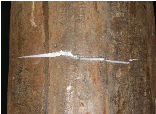
Pipe Rupture on Tension Surface – Slow Load Rate
